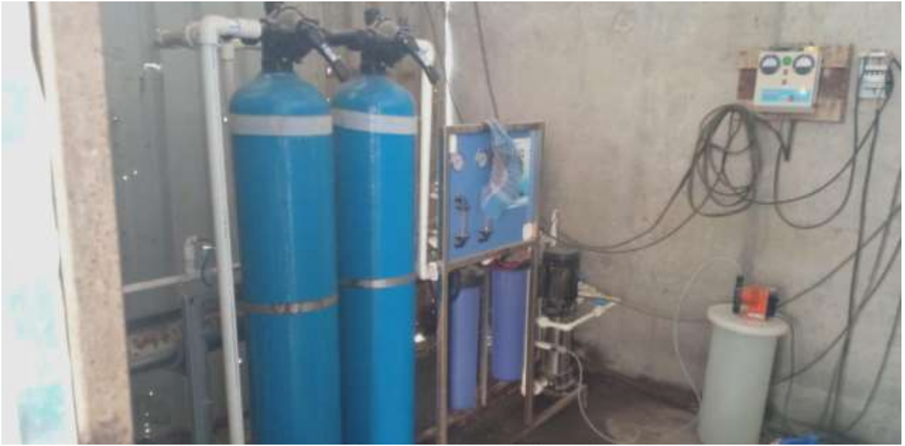
RO plant installed for drinking water
